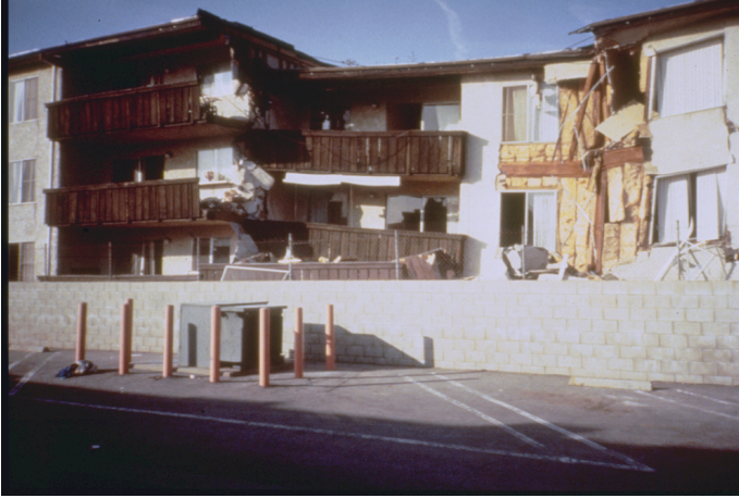
Figure 5.1 The Northridge Meadows Apartment Building where 16 people were killed in the 17 January Northridge earthquake. The apartment is located in an area of Northridge of about five square miles where intense damage occurred to this type of apartment. The building building had garages on the ends of the first floor and apartments in the middle. Some of these first floor apartments collapsed. (source: NOAA; photo: J. Dewey, USGS)
