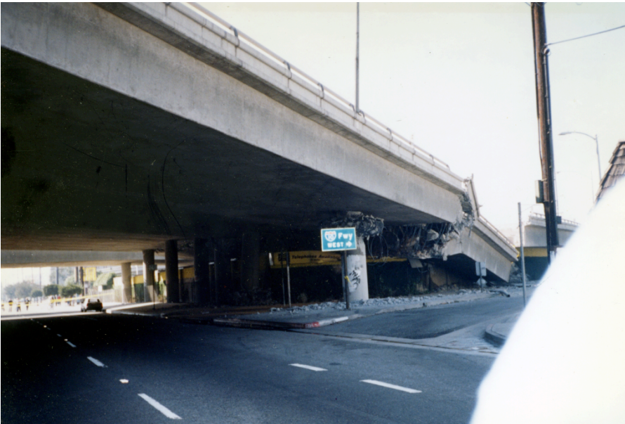
Figure 1.2 Collapsed section of the Santa Monica freeway (I-10) at La Cienega Blvd. exit after the 17 January 1994 Northridge earthquake. (source: Wikimedia)
